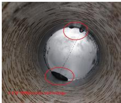
3-1/8"5000psi seat leakage
