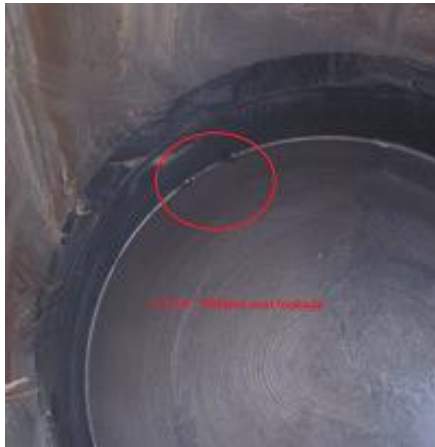
7-1/16"3000psi seat testing leakage
